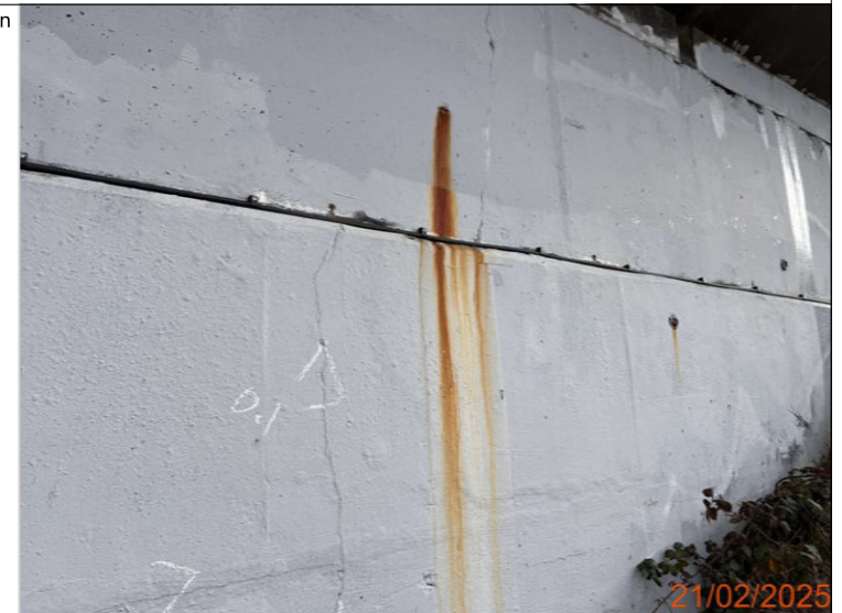
Rust staining to the south return wall on the east bankseat.JPG
