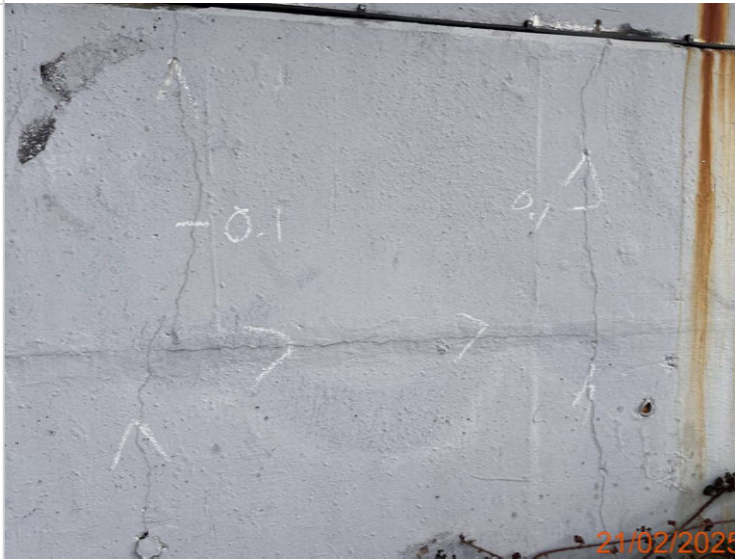
Cracking 0.1mm wide to the south return on the east bankseat.JPG
