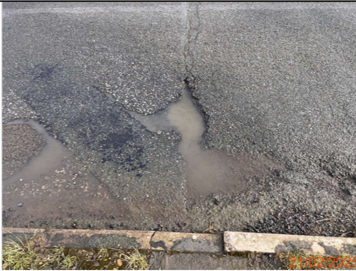
Pothole adjacent the east joint - 120 x 530 x 30mm.JPG
