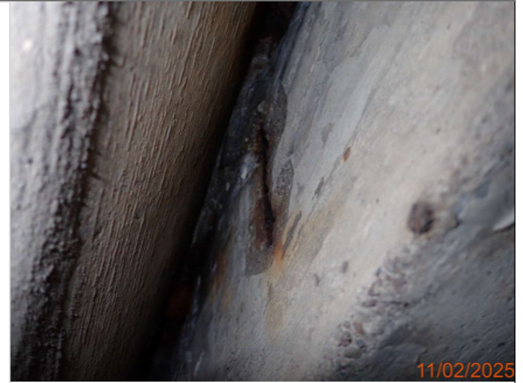
Spalling to the outer east hinge joint.JPG
