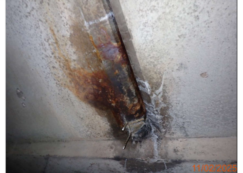
Rust staining to the south service bay over NB L1.JPG
