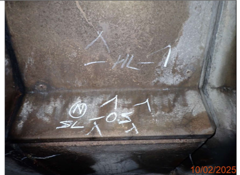
Cracking to the north service bay up to 0.5mm wide over NB L1.JPG
