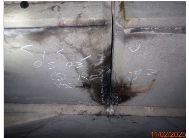
Cracking to the south service bay up to 0.5mm wide over SB HS.JPG
