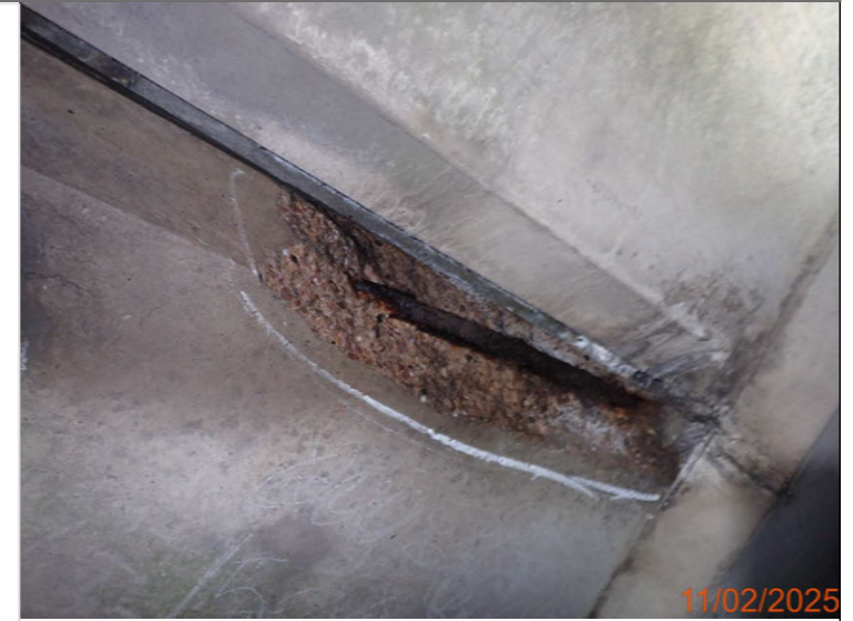
Spalling to the south service bay over SB L3 - 540 x 100 x 120mm.JPG
