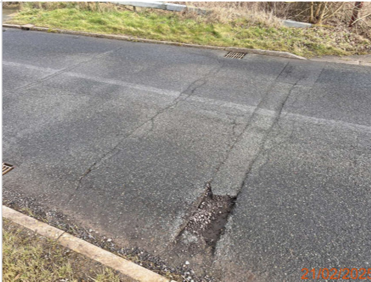
Pothole and transverse cracking on the east approach - 300 x 600 x 50mm.JPG
