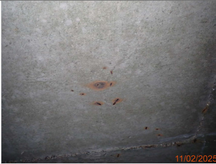
Rusty tie wire to the west span soffit.JPG
