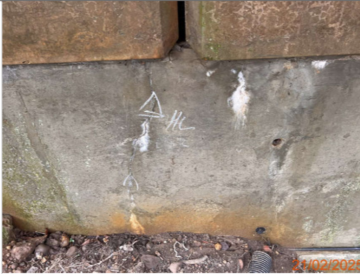
Hairline cracking to the north return on the east bankseat.JPG
