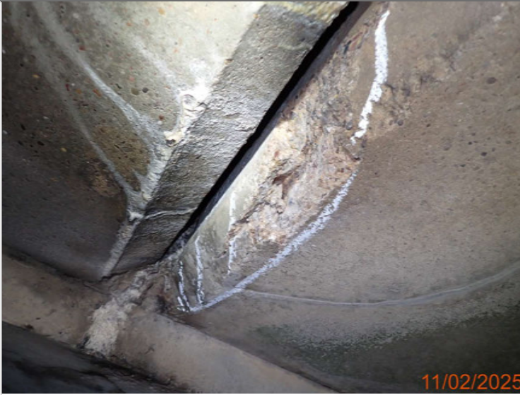
Spalling and delamination to the south service bay over SB slip - 530 x 140 x 50mm.JPG
