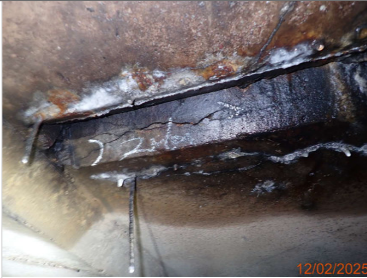
Cracking 2mm wide to the north service bay over NB L3.JPG
