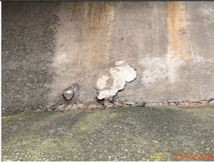
Minor delamination to the west bankseat.JPG
