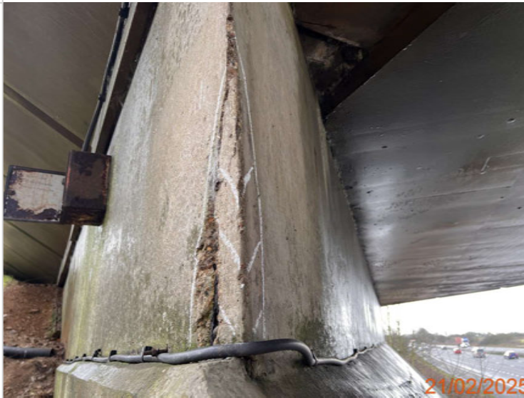
Delamination to the north end of the east bankseat - 190 x 430 x 20mm.JPG
