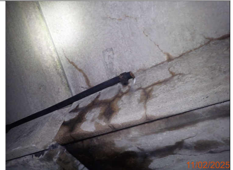
Hairline cracking to the north service bay over SB L1.JPG
