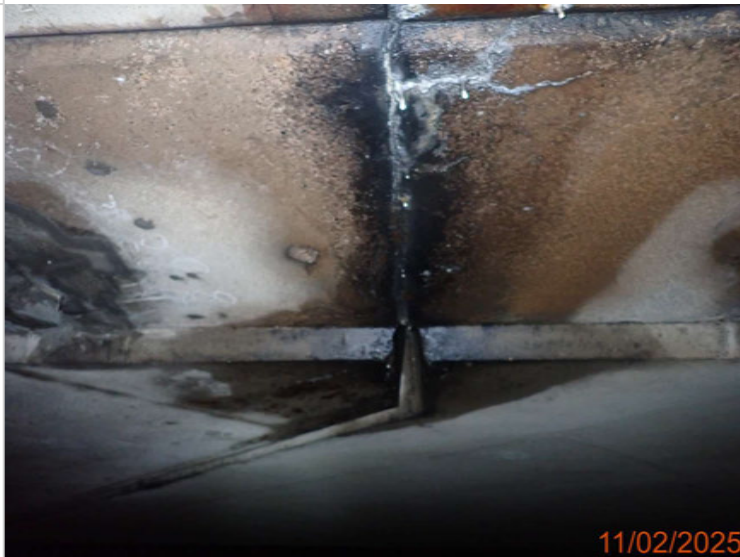
Water seepage through the east deck west hinge joint.JPG
