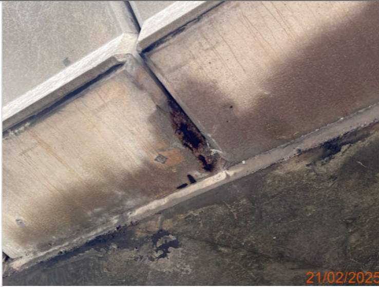
Spalling to the south service bay within the east span soffit.JPG
