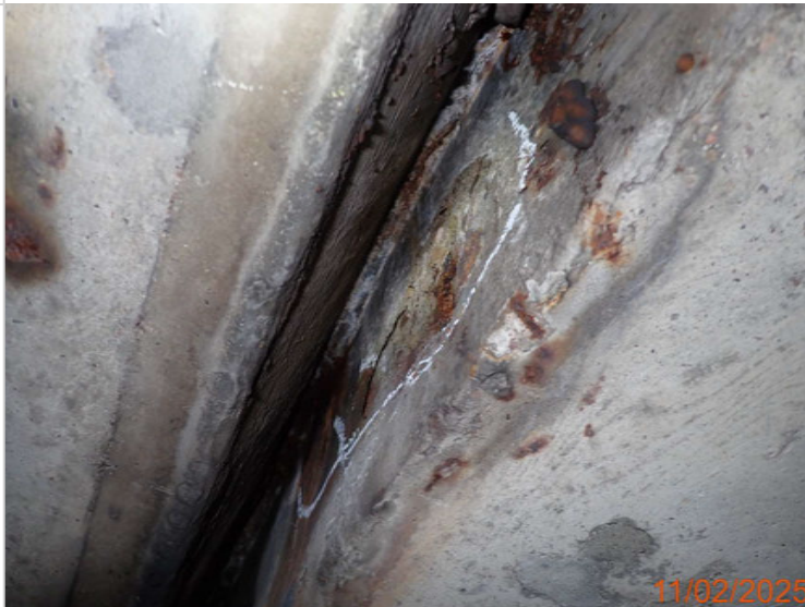
Spalling and delamination to the east outer hinge joint - 430 x 240 x 10mm.JPG
