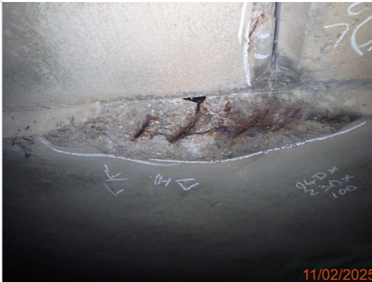
Spalling to the deck soffit over SB L2 - 940 x 230 x 100mm.JPG
