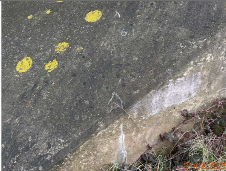
Cracking 0.1mm wide to the east revetment.JPG
