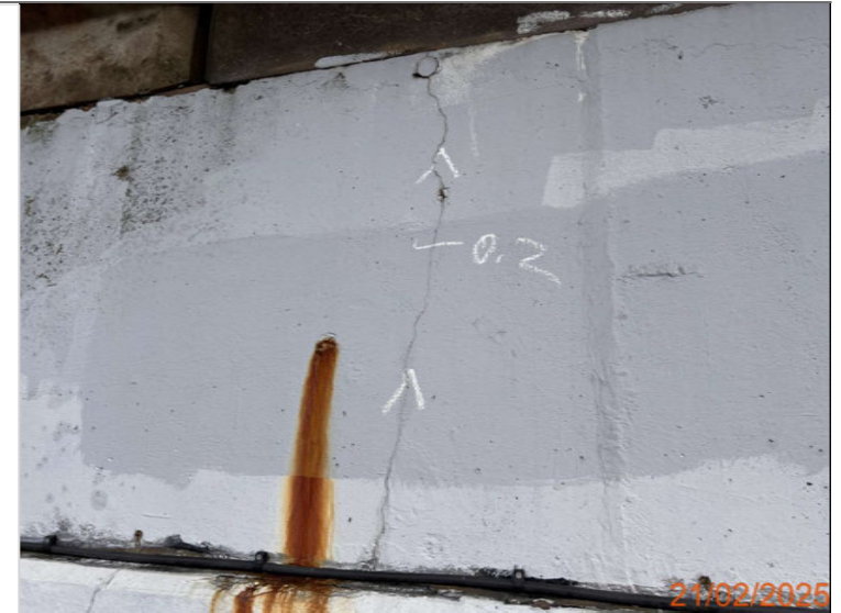
Cracking 0.2mm wide to the south return on the east bankseat.JPG
