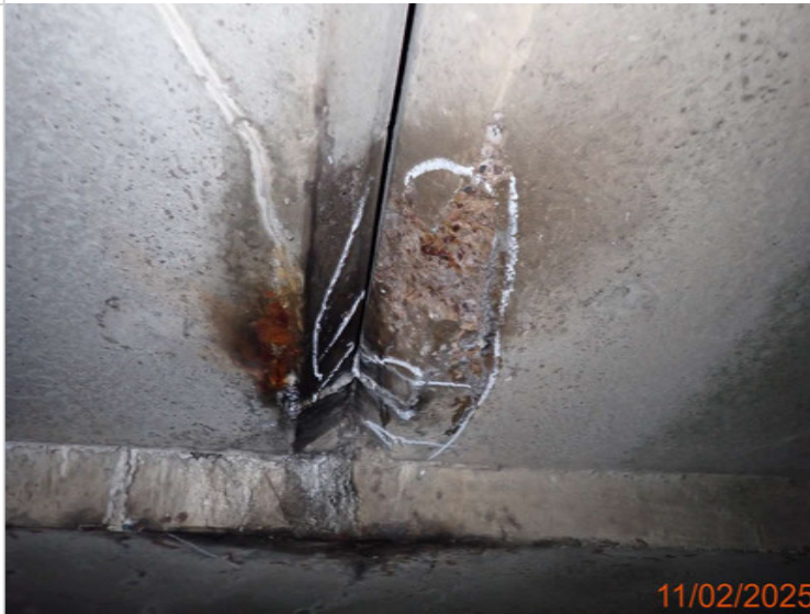
Spalling to the south service bay over NB slip - 440 x 170 x 20mm.JPG
