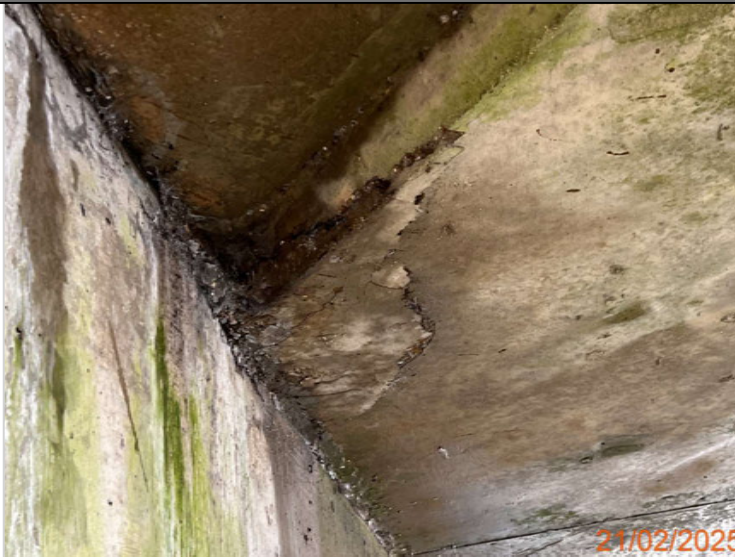
Delamination to the west span soffit adjacent the bankseat - 750 x 800mm approx.JPG
