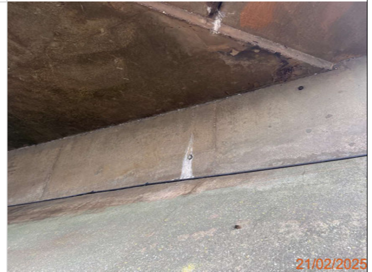
Vertical cracking to the east bankseat at the south end.JPG
