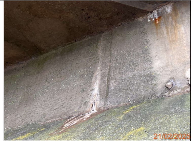
Vertical cracking to the west bankseat at the north end.JPG
