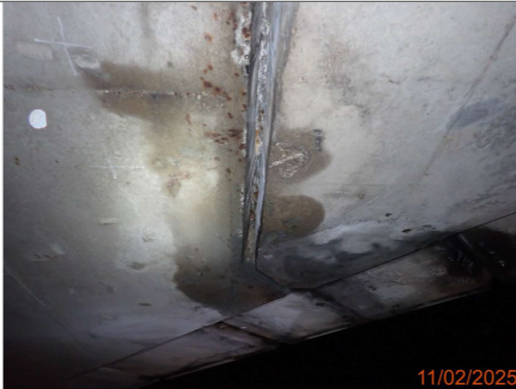
Water seepage through the east deck west hinge joint on the north end.JPG
