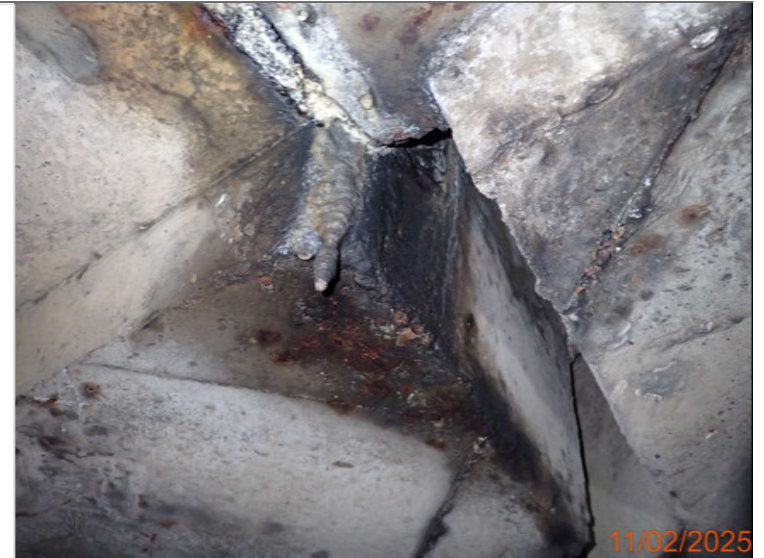
Water seepage through the south end of the west hinge joint.JPG
