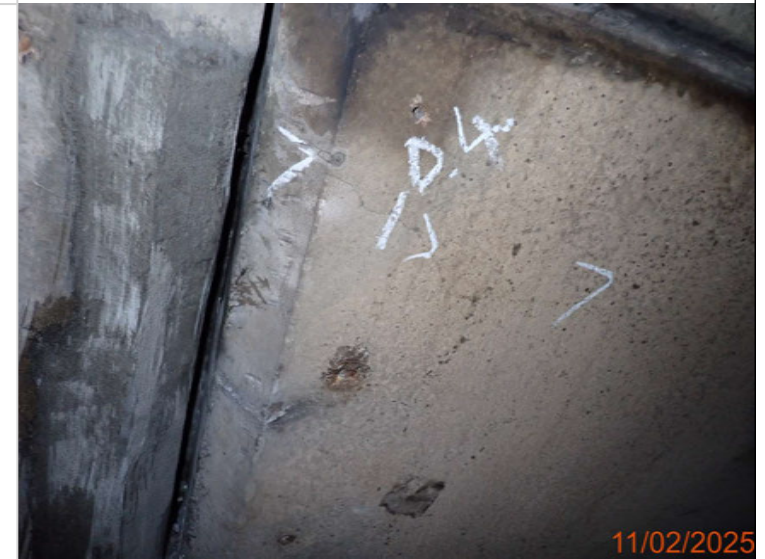
Cracking to the south service bay 0.4mm wide over NB L1.JPG
