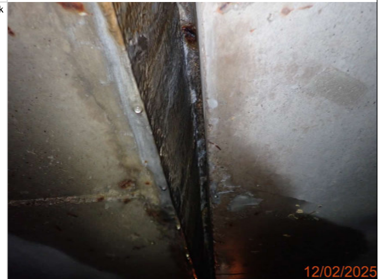
Leachate through the west deck east hinge joint.JPG
