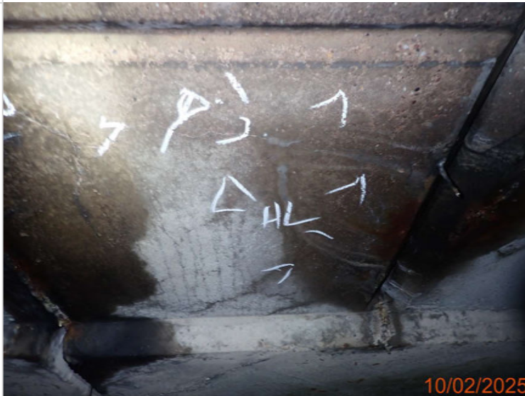
Hairline cracking to the north service bays over NB L1.JPG
