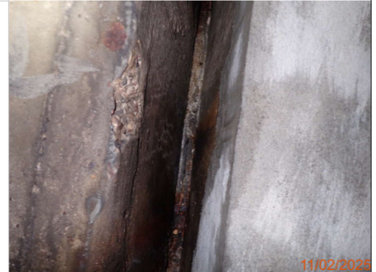
Cracking within the east hinge joint over SB L1.JPG
