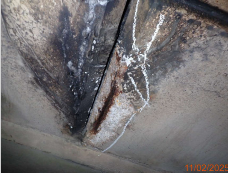
Spalling and delamination to the south service bay over SB L1 - 850 x 210 x 180mm.JPG
