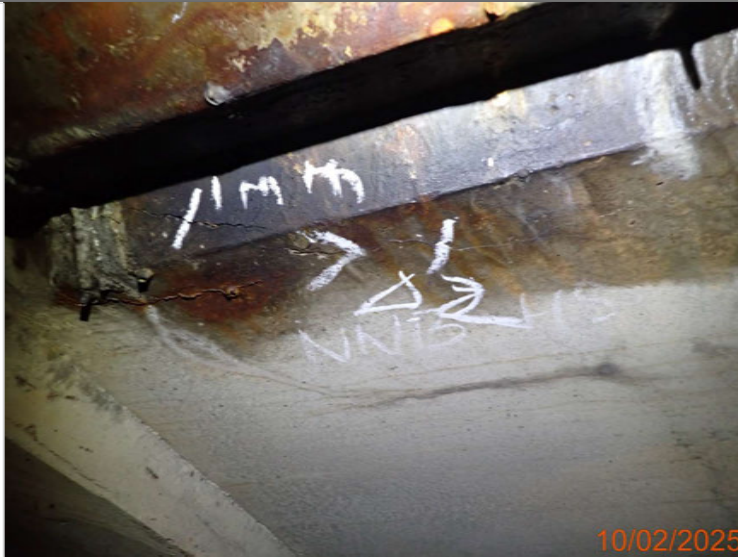
Cracking 1mm wide to the north service bay over NB L1.JPG
