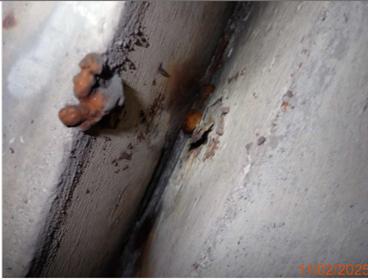
Minor spalling to the east outer hinge joint.JPG
