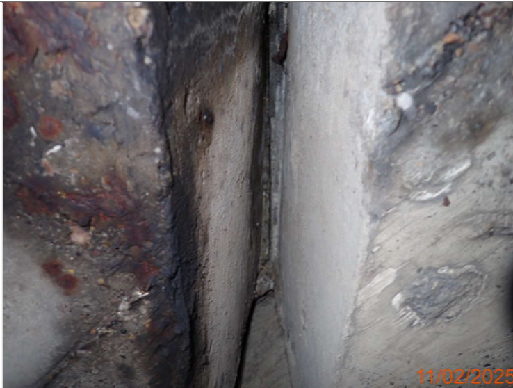
Cracking within the west hinge joint over NB L1.JPG
