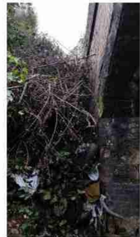
Plate 3 Arch 3 infilled on both sides but with a narrow bat accessible gap on the north west facing side leading into a large internal void (Not visible in photo)
