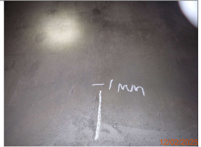
Vertical cracking 1mm wide to the west face of the centre pier.JPG
