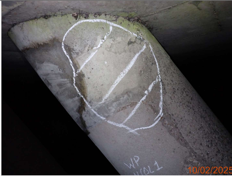
Delamination to the upper column 1 on the west pier - 400 x 530mm.JPG
