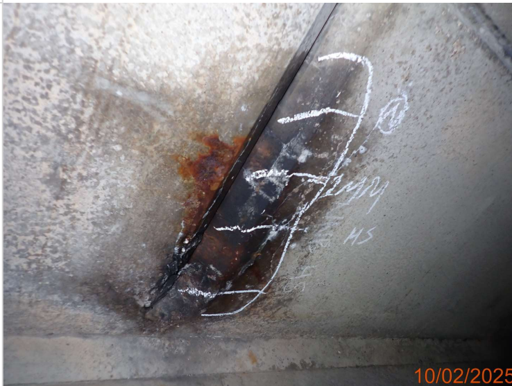
Delamination to the north service bay over NB L1 - 690 x 220mm.JPG
