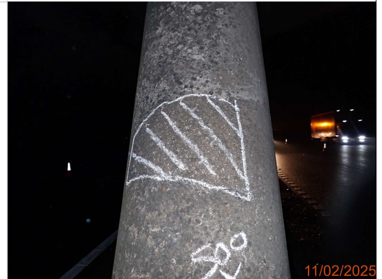
Delamination to the south end of the centre pier - 500 x 370mm.JPG
