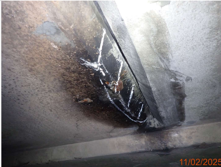
Delamination to the south service bay over SB L1 - 510 x 120mm.JPG
