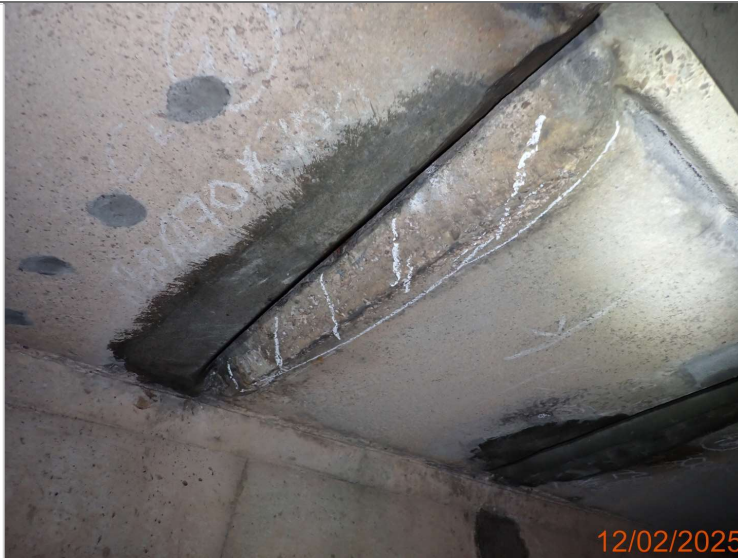
Delamination to the south service bay over NB L3 - 840 x 160mm.JPG
