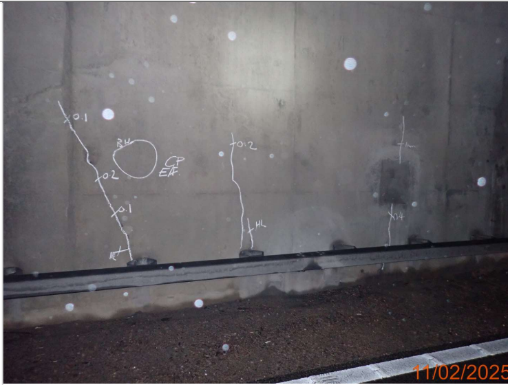
Cracking to the east face of the centre pier up to 1mm wide.JPG
