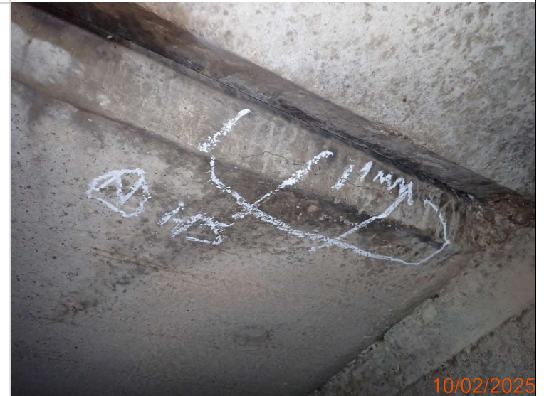
Delamination to the north service bay over NB L1 - 400 x 150mm.JPG
