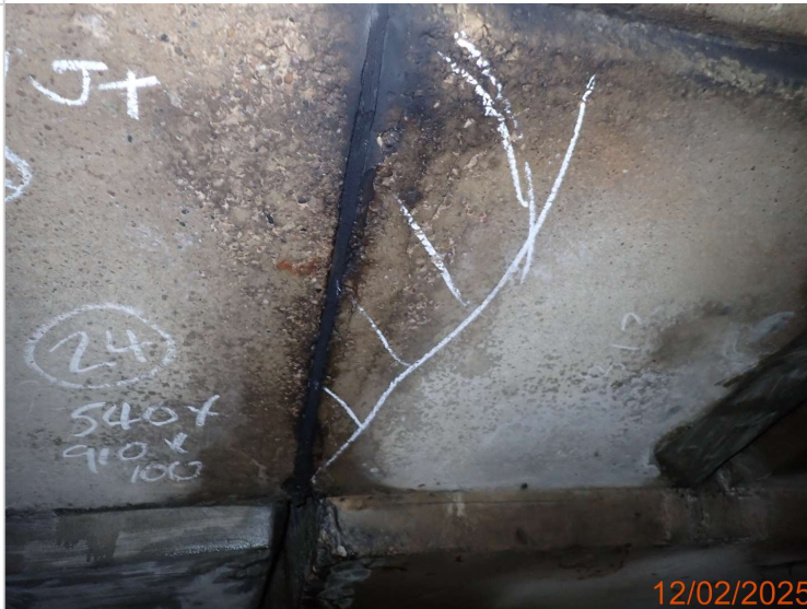
Delamination to the south service bay on the outer west hinge joint over NB L3 - 850 x 200mm.JPG
