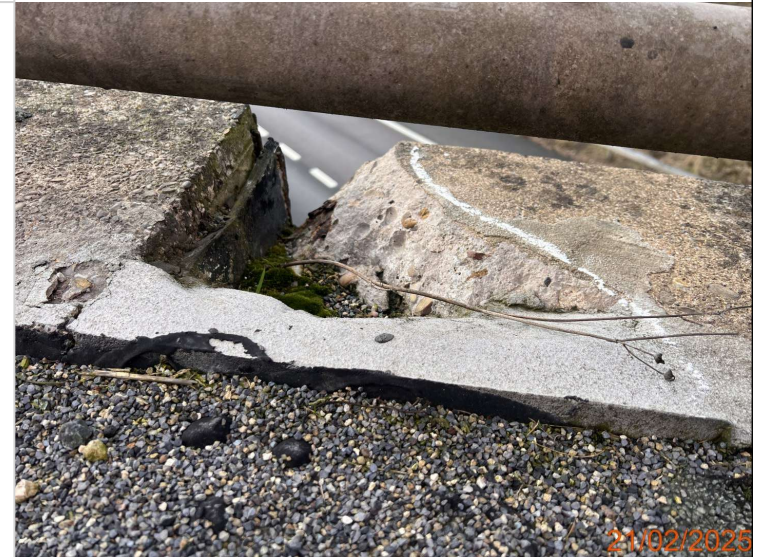
Spalling to the upper service bay over NB L3 - 350 x 240 x 70m.JPG
