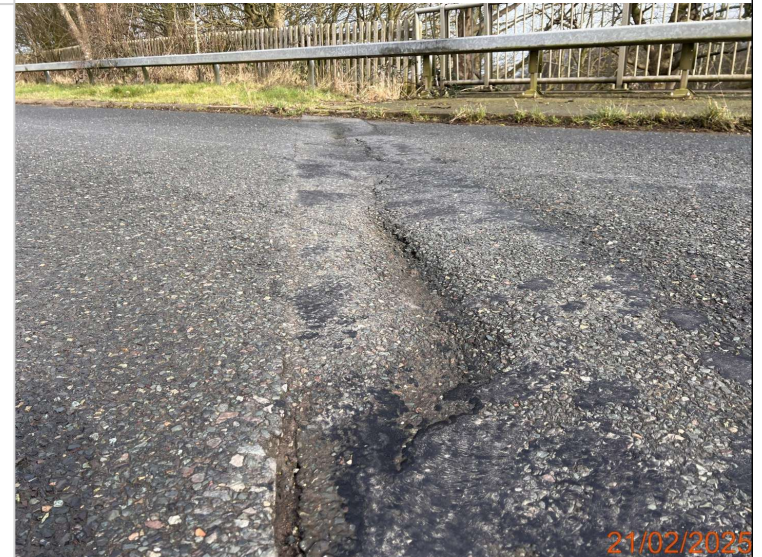
Settlement and cracking on the west joint.JPG
