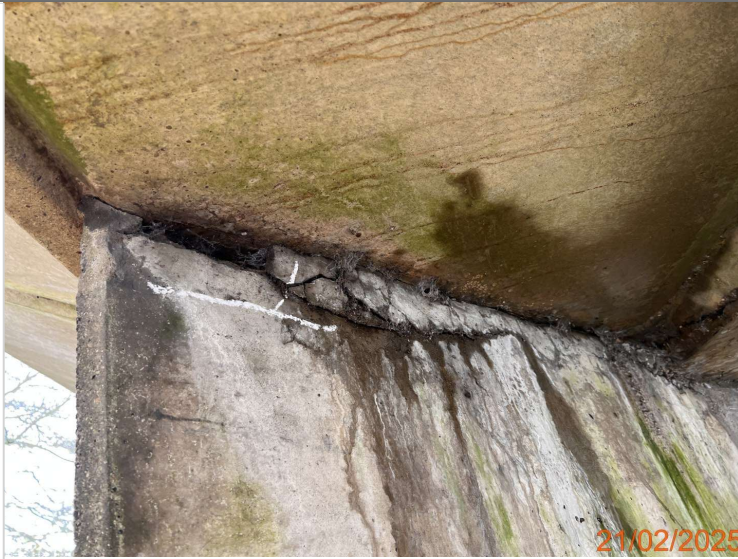
Delamination to the west bankseat - 730 x 110 x 10mm.JPG
