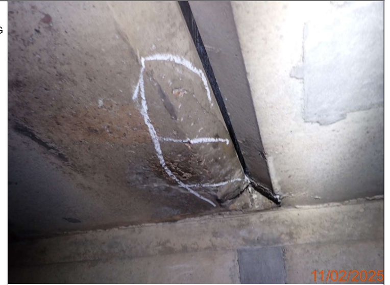
Delamination to the north service bay over the centre reservation - 510 x 160mm.JPG
