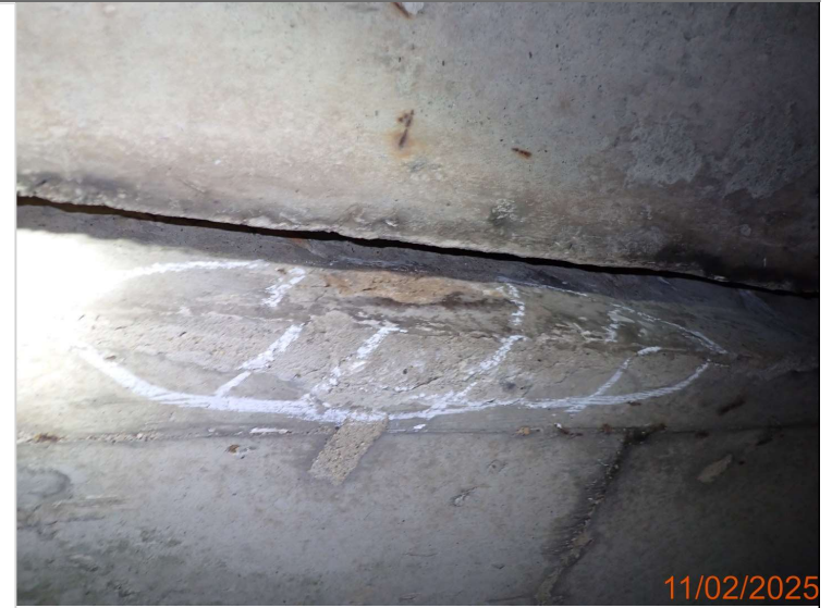
Delamination to the west hinge joint over the slip - 200 x 600mm.JPG
