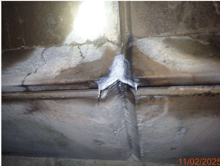
Leachate emanating between service bays over NB L1.JPG
